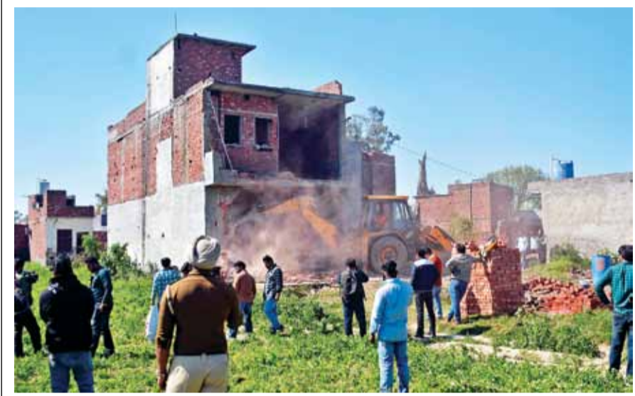
A house belonging to alleged drug peddler being bulldozed in Bhararawal area, in Amritsar on Thursday, March 06, 2025. In a major crackdown on drug trafficking, the Punjab government has demolished properties linked to drug traffickers in Amritsar, reinforcing its commitment to making the state drug-free. PHOTO-PRABHJOT GILL
